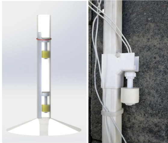
Figure 7 Float level reed sensors installation
