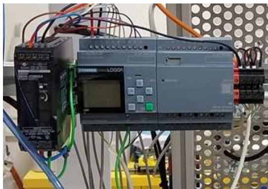
Figure 8 PLC control unit with expansion module in SIEMENS LOGO! v. 8.4 version
